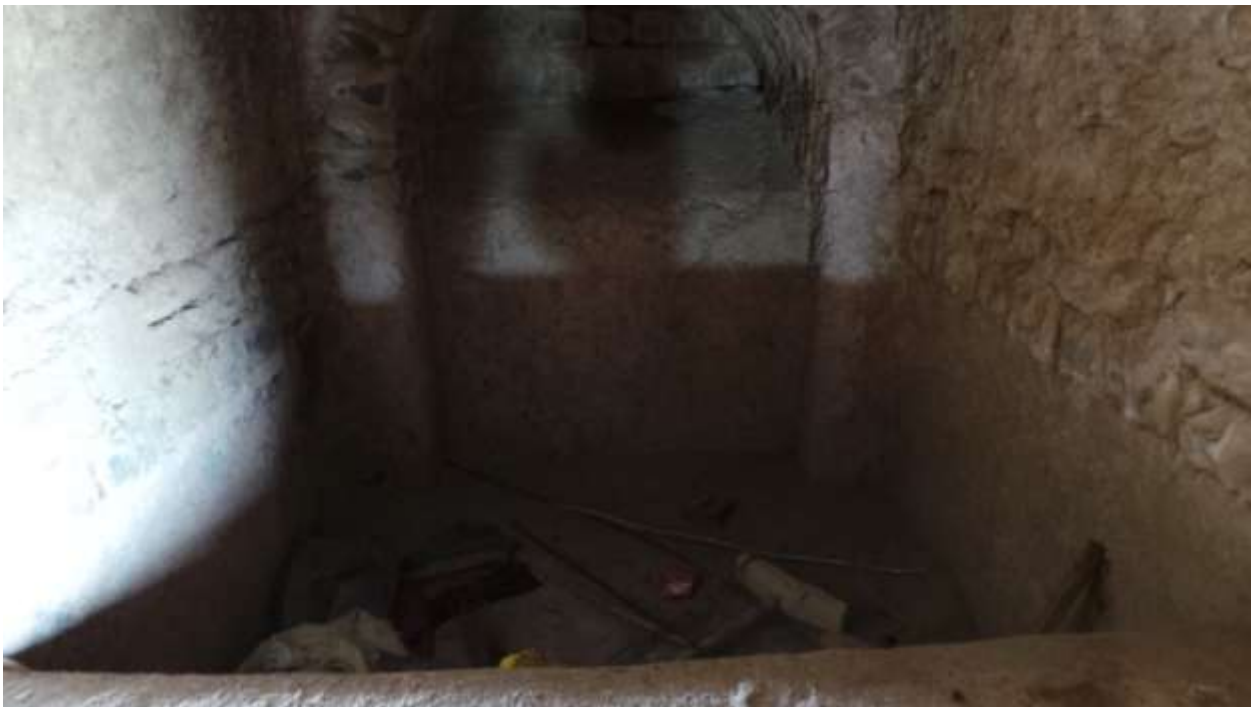
Plate 73- the smaller tank to which are connected the pipes that carry water from the terrace
