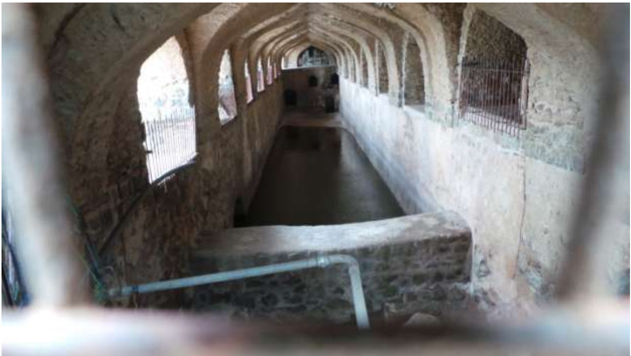
Eastern wall of the tank which is connected to the smaller tank
