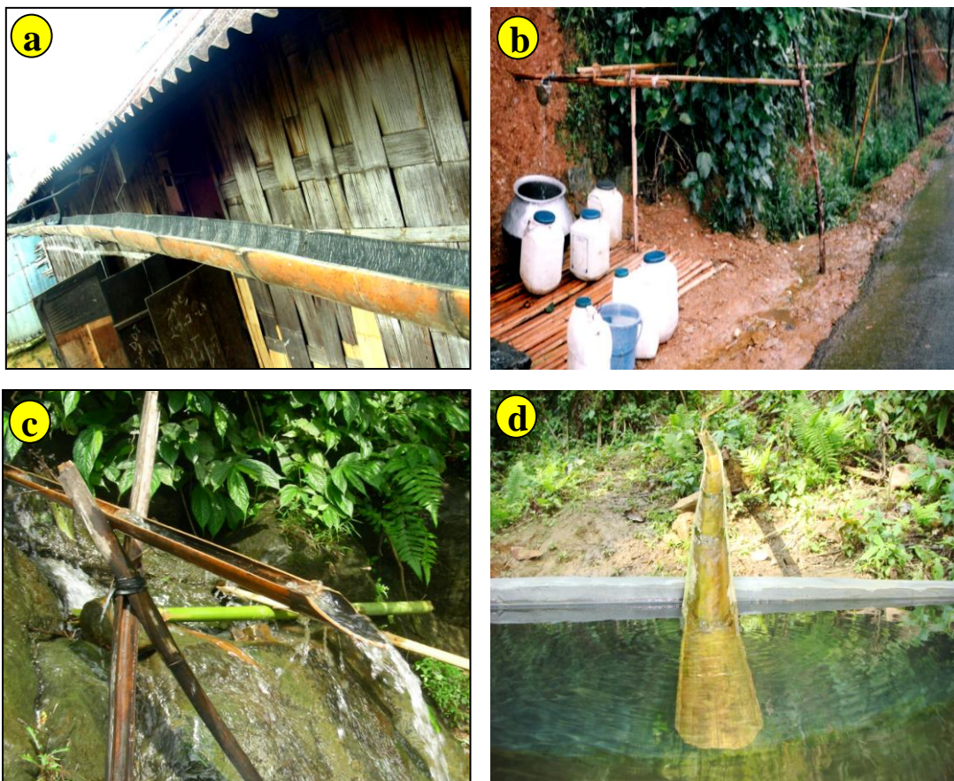
Figure 72. Bamboo pipes. a) Pipe for rain water collection from the roof top; b) Collection of water to their door step; c) Collection of water from the running river; d) Collection of water to the reservoir from the river source
